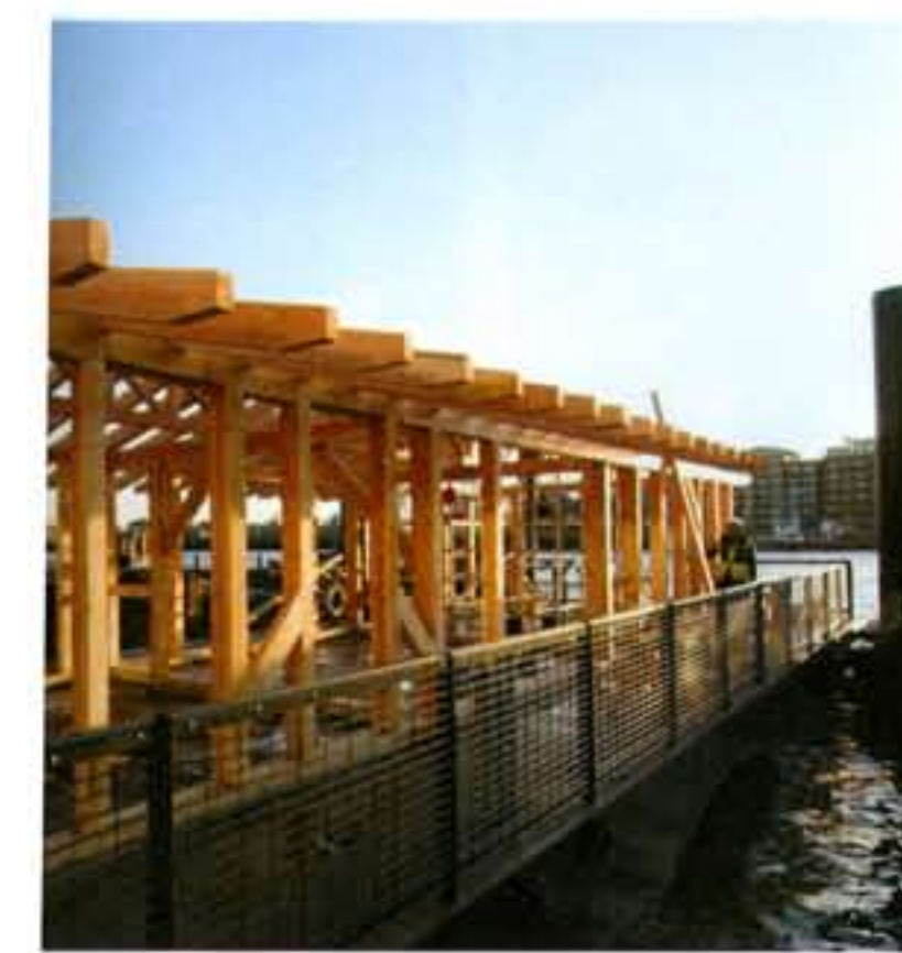
Left: the pier house at high tide. The pontoon rises and falls with the Thames 7m a day
