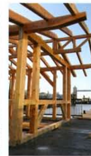
Above: a Howe truss runs the length of the building. The entire frame is in west country Douglas fir from Pennymoor Timber of Tiverton
